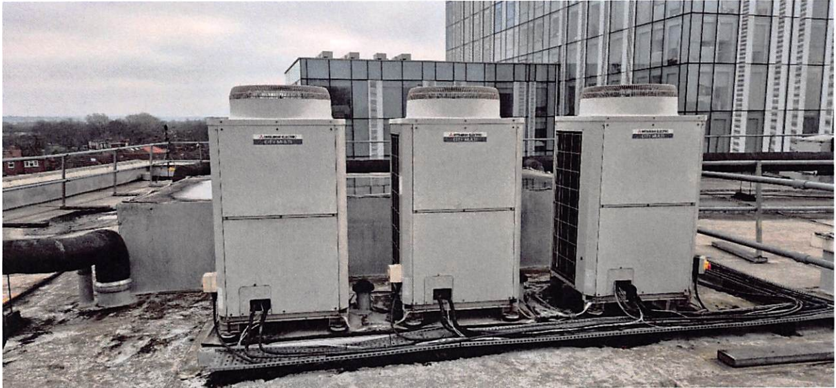
Figure D9 – Photograph of 3no. Mitsubishi 'CITY MULTI' Air Conditioning units (PURY-P200YJM-A), located on existing hotel roof (17 m west of Position 1, visible in background of photograph).
