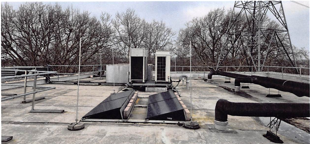
Figure D10 – Photograph of 4no. Mitsubishi 'CITY MULTI' Air Conditioning units (PURY-P200YJM-A), located on existing hotel roof (33 m west of Position 1).
